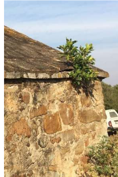
Right: Ficus sapling growing out of roof (Photo: Tom Barrett)
